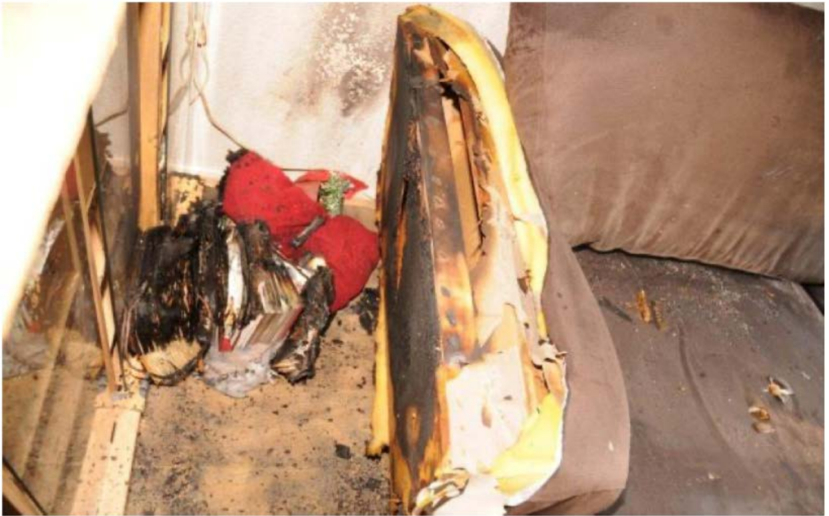
Foto 9: Secondaire brand woning 1 e verdieping
